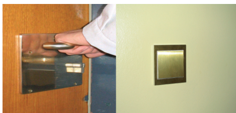
Fig 2: First products installed in a hospital for approval
